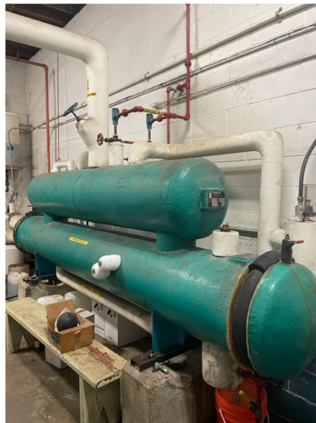
Fig. 1 – NGCC Chiller in the ice plant / compressor room
